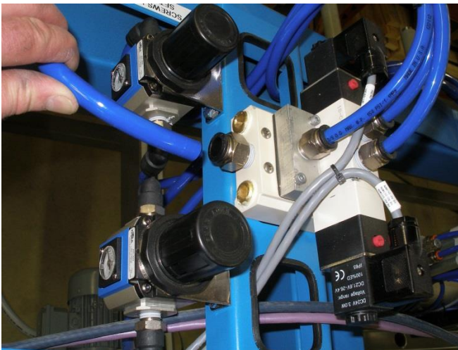
Airline connection on Gantry
