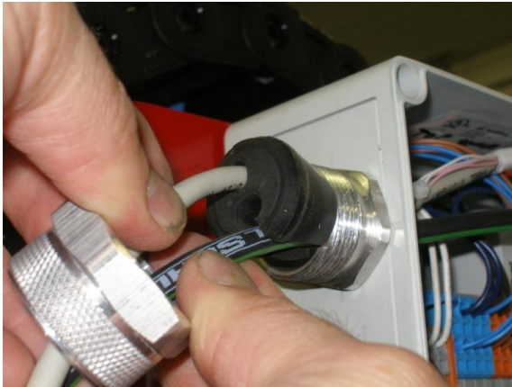
Ethernet Cable routing – Gantry Enclosure
