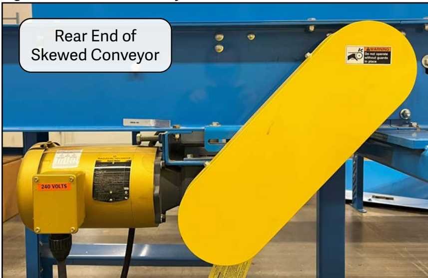
Figure 7-43: Skewed Conveyor Chain Lubrication Point
