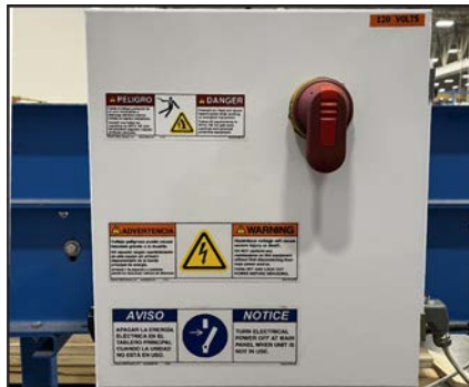
Skewed Conveyor Disconnect Switch
