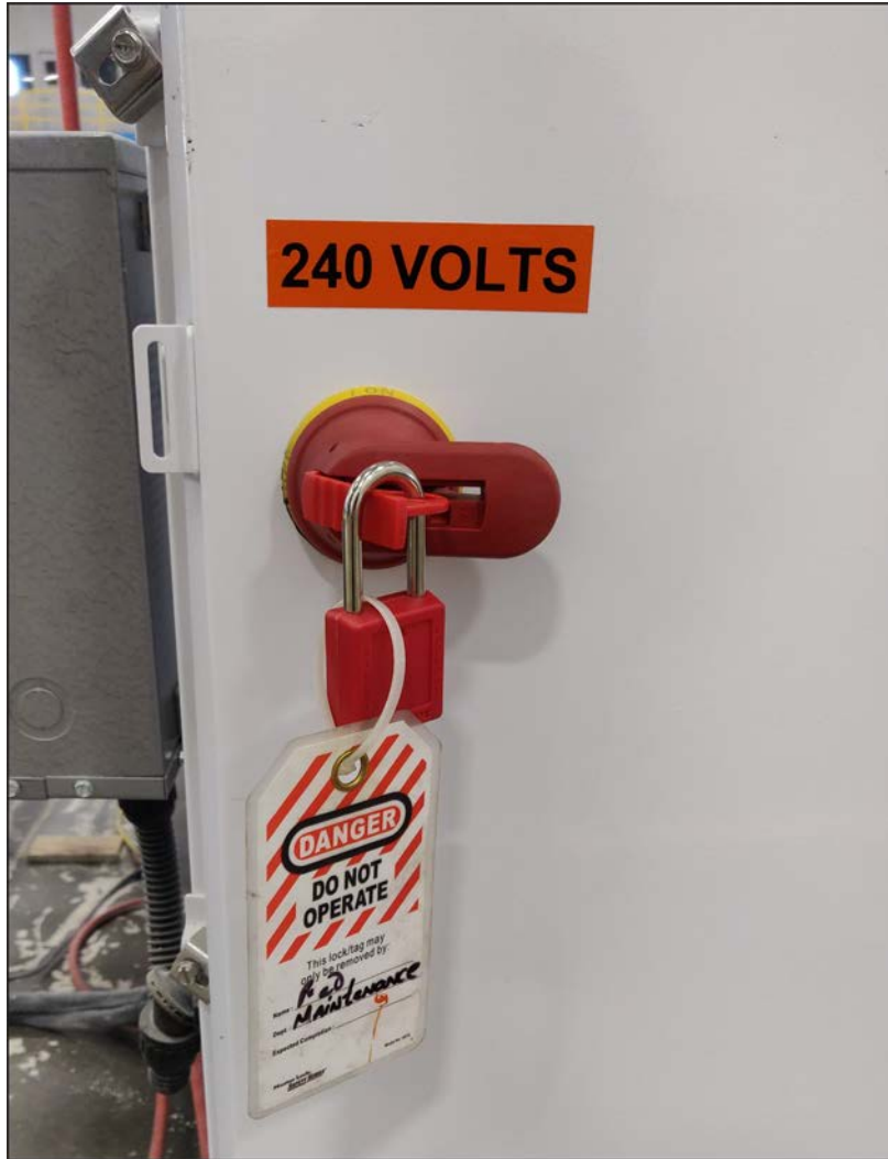
Figure 1-2: Sample of a Lockout/Tagout Mechanism on an Electrical Enclosure
