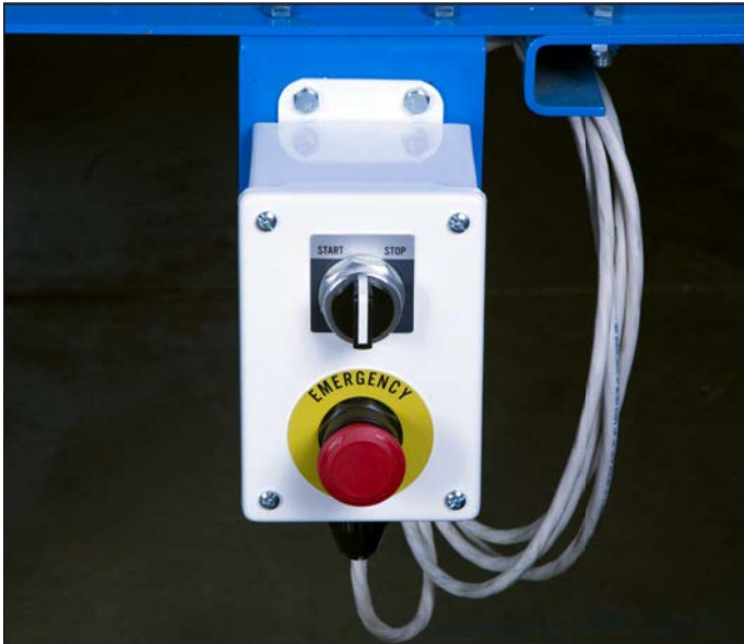
Figure 6-9: Skewed Conveyor Controls
