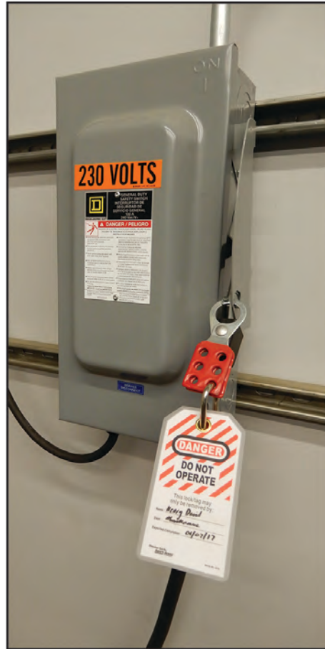
Figure SAFETY-5: Sample of a Lockout/Tagout Mechanism on a Power Source Panel
