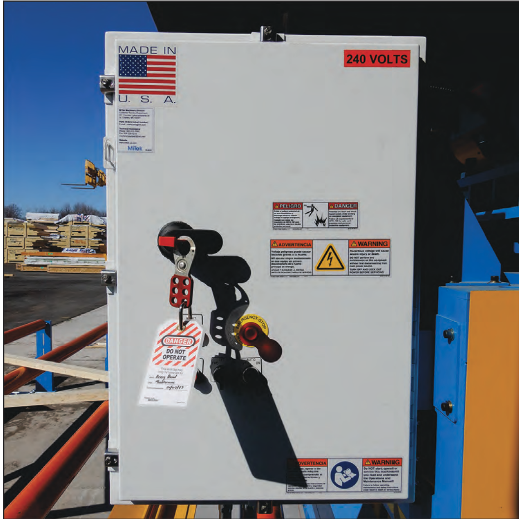
Figure SAFETY-4: Sample of a Lockout/Tagout Mechanism on an Electrical Enclosure
