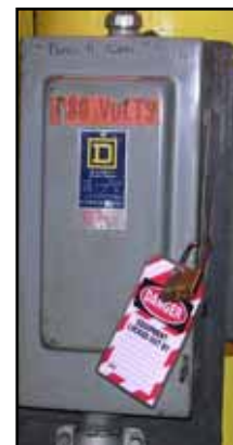
Figure 1: Lockout/Tagout on the Power Source Panel
