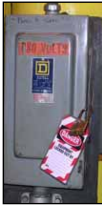
Figure 2: Lockout/Tagout on the Power Source Panel
