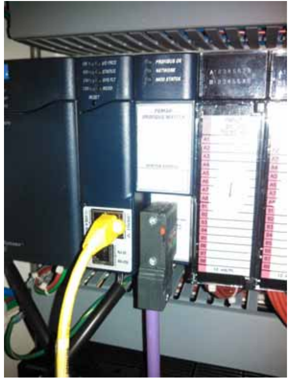
Figure 16: Ethernet and Profibus Cables
