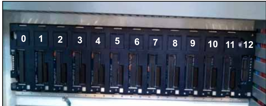
Figure 11: The New Backplane Installed, With Slots Numbered
