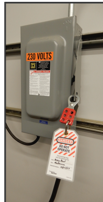
Figure 1: Lockout/Tagout on the Power Source Panel
