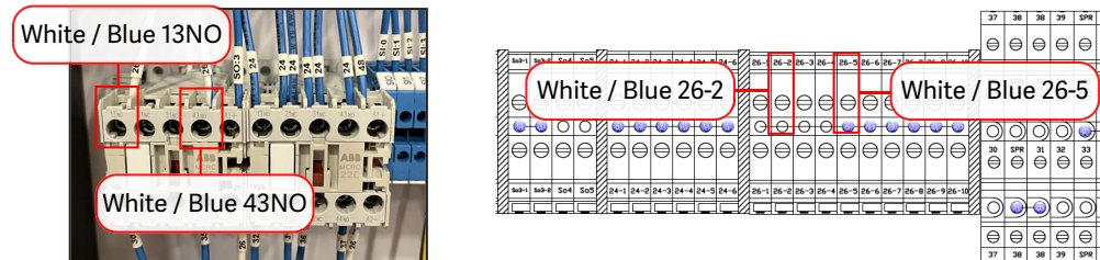
Figure 18: Existing Wires to Remove at CR2 (labeled in enclosure)
