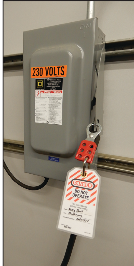
Figure SAFETY-4: Sample of a Lockout/Tagout Mechanism on a Power Source Panel
