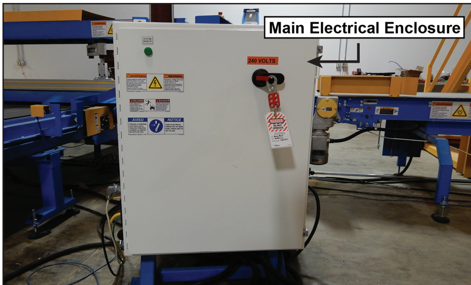
Figure SAFETY-3: Main Electrical Enclosure with Lock and Tag
