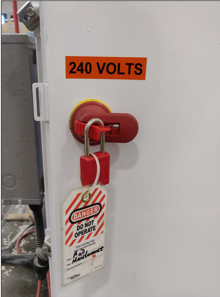
Figure 1-2: Sample of a Lockout/Tagout Mechanism on an Electrical Enclosure
