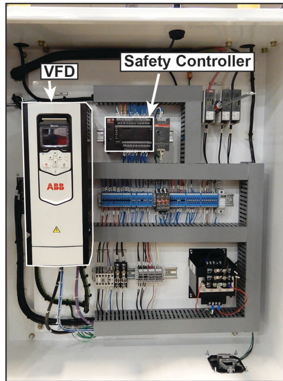
Figure 6-3: Main Electrical Enclosure
