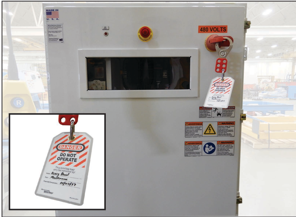
Figure SAFETY-1: Lockout/Tagout Mechanism on Main Electrical Enclosure
