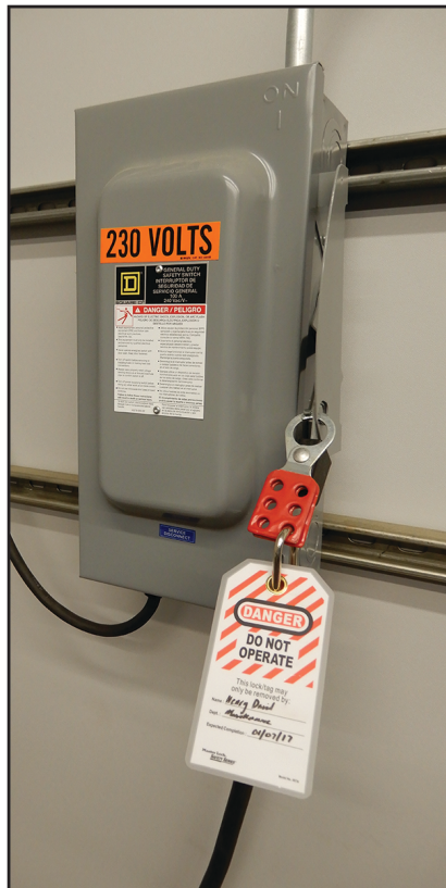
Figure SAFETY-2: Sample of a Lockout/Tagout Mechanism on an Electrical Service Entry Panel
