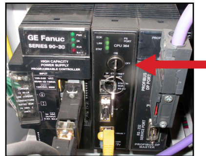
Figure 2-70: Turn Key TWICE to Reset the PLC
