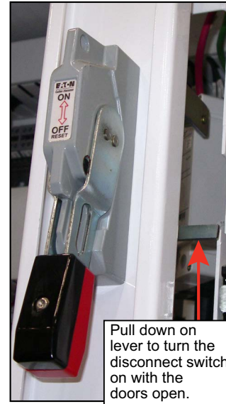
Figure 2-69: Turning On the Disconnect Switch
