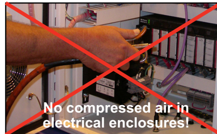
Figure 2-19: Never Use Compressed Air Inside an Electrical Enclosure
