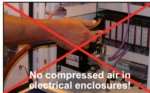
Figure 6-7: Never Use Compressed Air Inside an Electrical Enclosure
