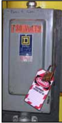
Figure 1: Lockout/Tagout on the Power Source Panel
