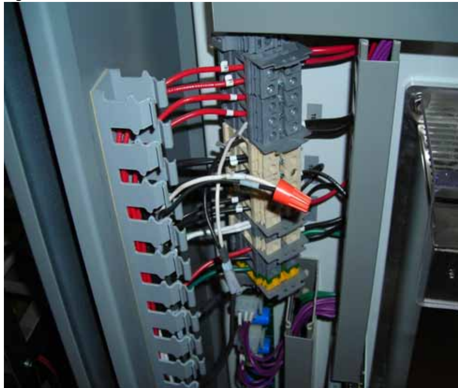
Figure 2: TB1 and TB2 Terminal Blocks in the AC Power Box
