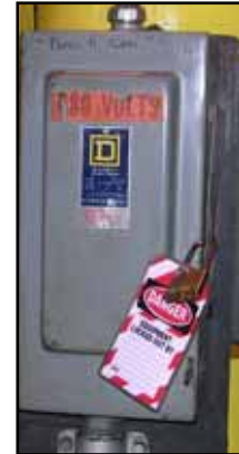
Figure 1: Sample of Lockout/Tagout on a Power Source Panel
