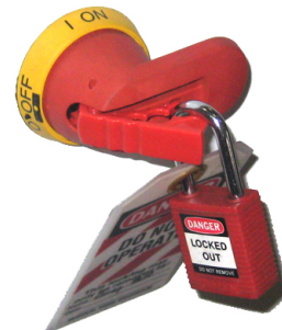
Figure 1: Lockout/Tagout on the Main Electrical Enclosure
