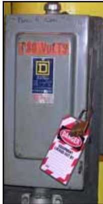
Figure SAFETY-3: Sample of a Lockout/Tagout Mechanism on a Power Source Panel
