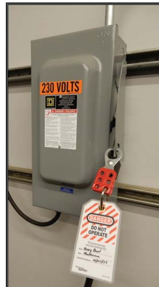
Figure 1: Lockout/Tagout on the Power Source Panel
