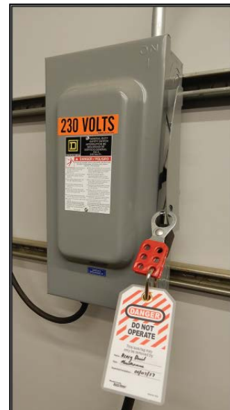
Figure 1: Lockout/Tagout on the Power Source Panel
